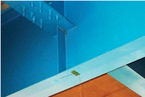
Fig. 5. Welding of a vertical stiffener and bottom flange of a cross beam
